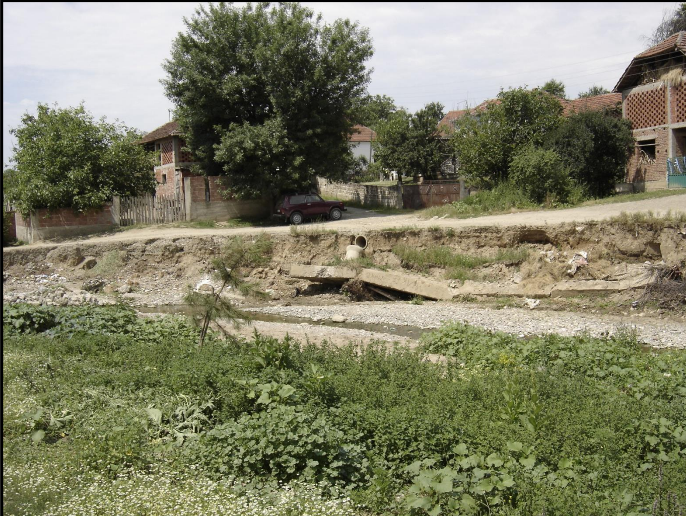
Destroyed retaining wall and sewerage outflow
