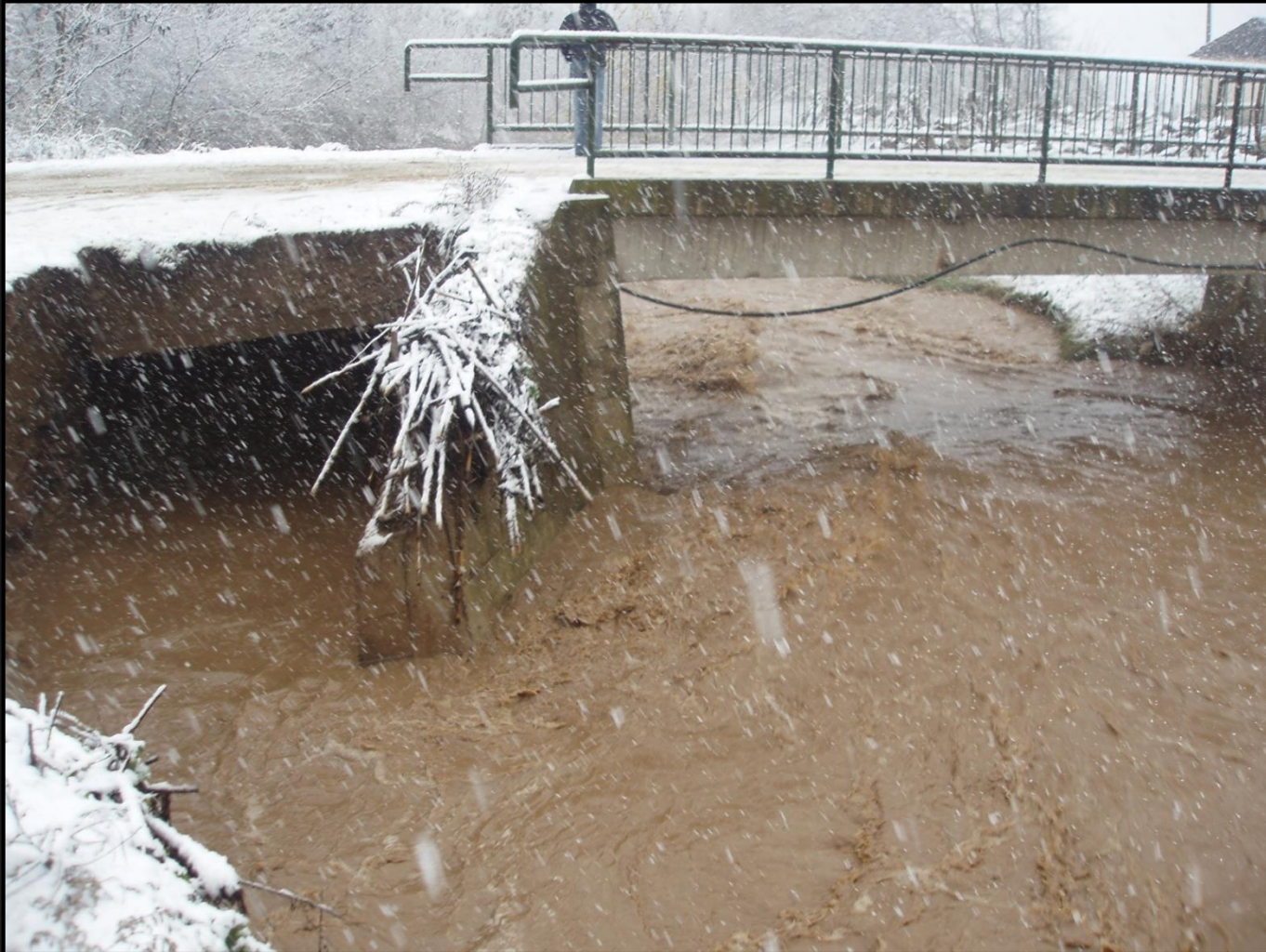
Endangered local bridge
