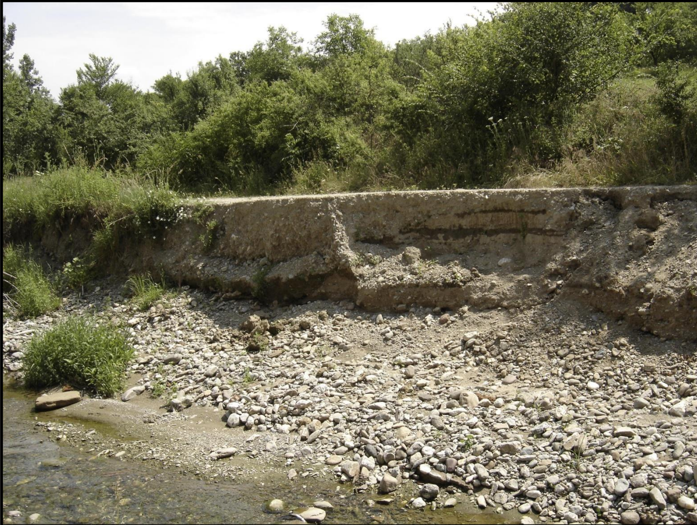
Destroyed local road (300m)
