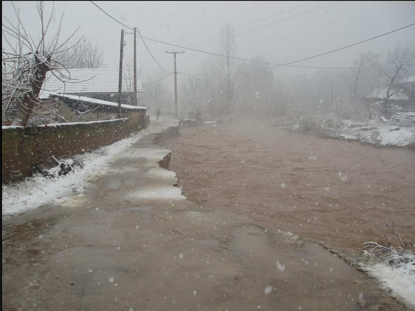
Destroyed local road (200m)
