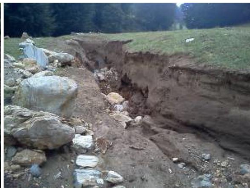
Figure 46 - Gully on the grassland (section 1-2)
