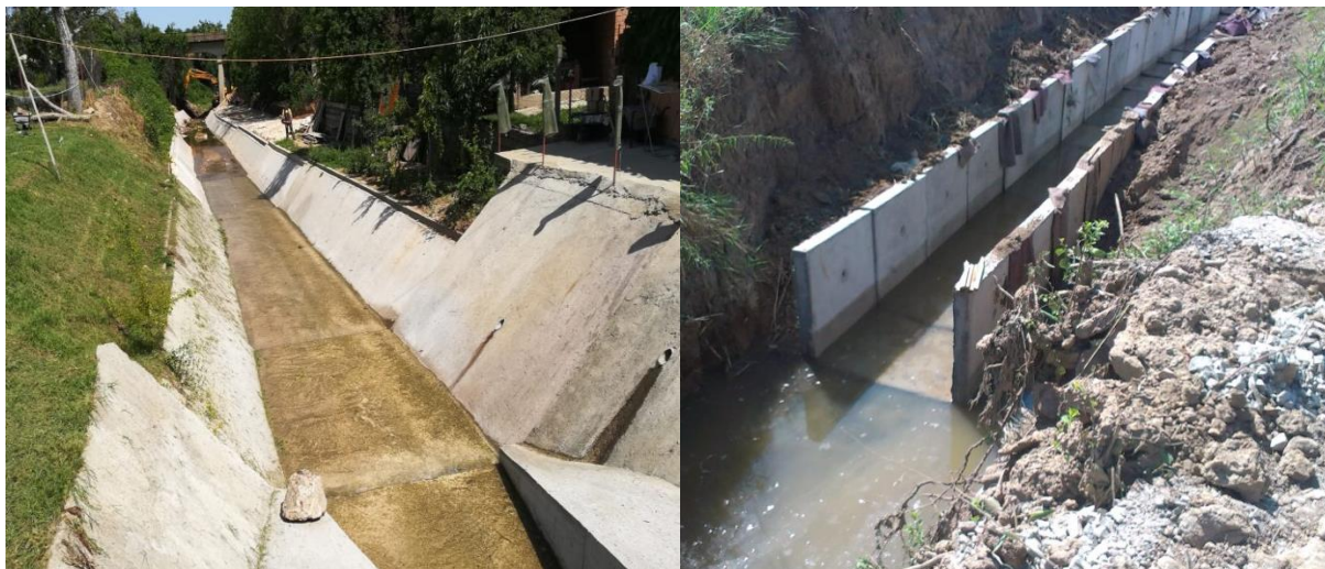
Figure 11. Regulation work on Rokov and Bukovac streams (north face of the Fruška Gora)
