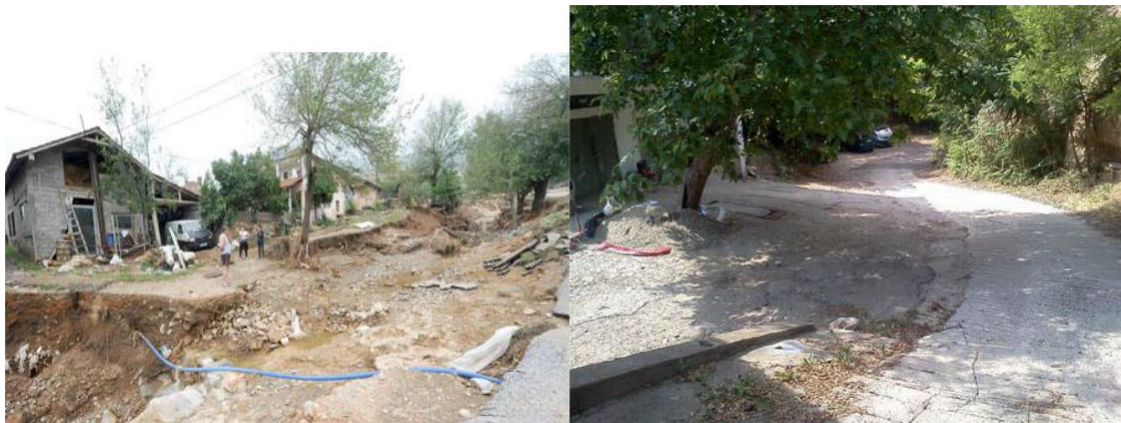
Figure 10 - Illegal dike for crossing and total covering of the bed and directing the water on the street
