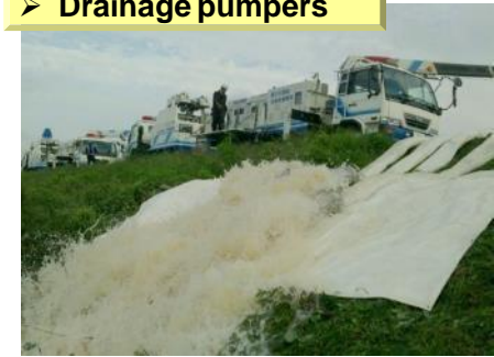
Torrential rain in Kanto and Tohoku (September 2015) (Kurihara City, Miyagi Prefecture)
